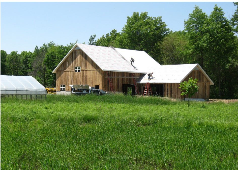
Construction workers install white metal roofing on the new barn at Rieth Village. This view is taken from Oshtemo Cottage, looking southwest.
